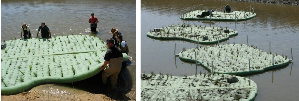
Figure 6a (left). Launching a floating wetland island. Figure 6b (right). Installing goose prevention fencing.
