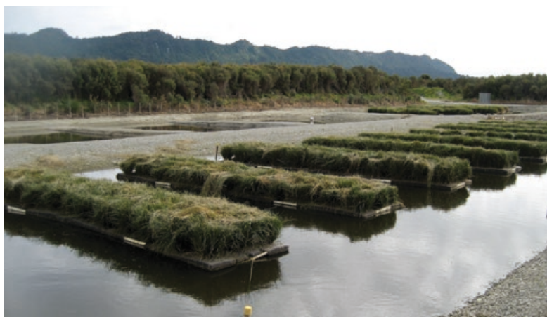
Treatment of landfill leachate using BioHaven® technology. McLeans Pit, Town of Greymouth, South Island, New Zealand. Image provided by Leela O’Dea.
